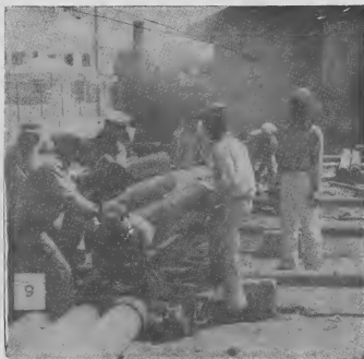
9 - A "side-line" job at the Salvage Yard is corrosion-proofing pipe for road underpasses. Made up in advance of need, a supply of sizes from 6 to 16 inches is kept on hand, to minimize the time a road may be blocked by excavation. Pipe is cleaned, coated with protective primer, coated with hot asphalt, wrapped in burlap, then coated again with asphalt. (The final operation is shown in the picture.)
